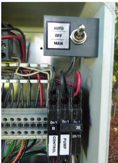
Figure 2 Typical pump controls (top) and circuit breakers (bottom) found inside control box.
