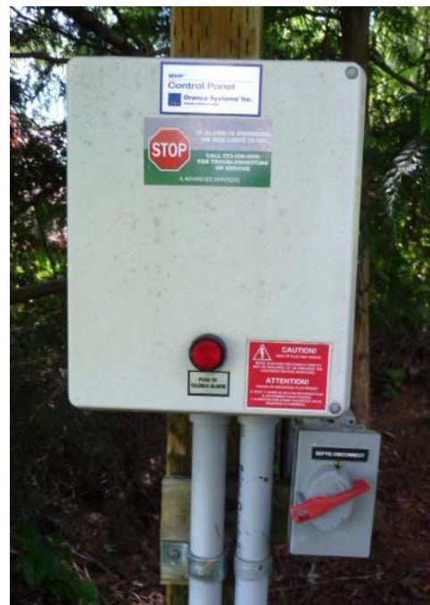
Figure 1 Typical septic tank control box with red indicator button (center) and main power switch (bottom right).
